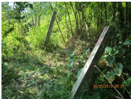
Figure-4. The condition of bars from T967-T972 which need to be repaired
