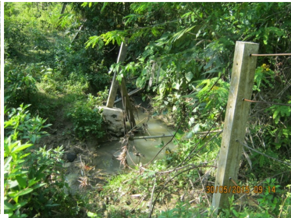
Figure-2. The condition of bars from T967-T972 which need to be repaired
