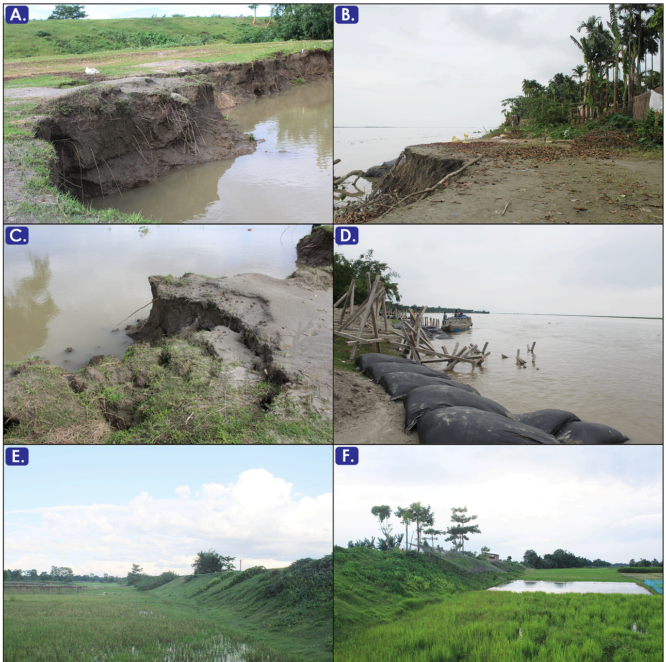
Fig. 7. A) to C) Erosion along the banks of the Brahmaputra D) Porcupines and geobags to protect banks from erosion E) and F) Embankments to secure banks from further erosion.
