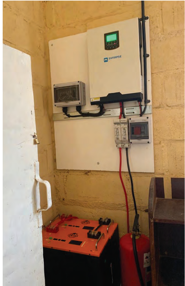
Solar panel electricity system
