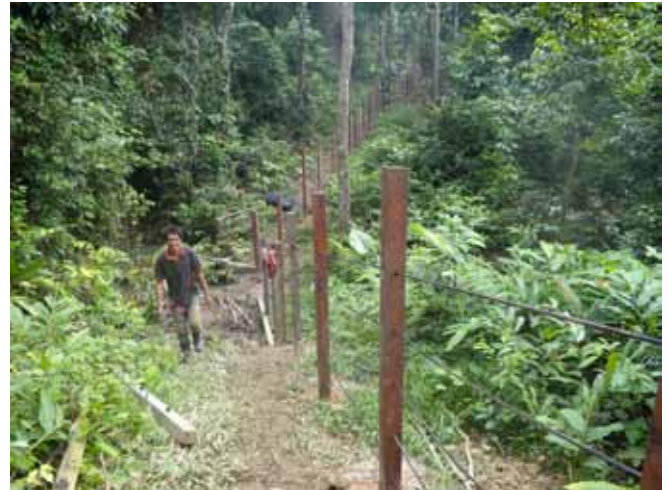
Construction of a temporary 2.5 hectare rhino paddock at Tabin, financed by Sabah Forestry Department.
