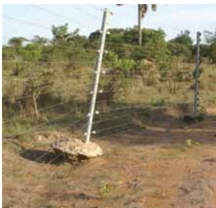
Soil erosion around fence posts.
