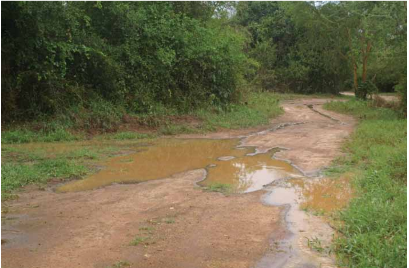
Problems of water-logging and road erosion were prevalent.
